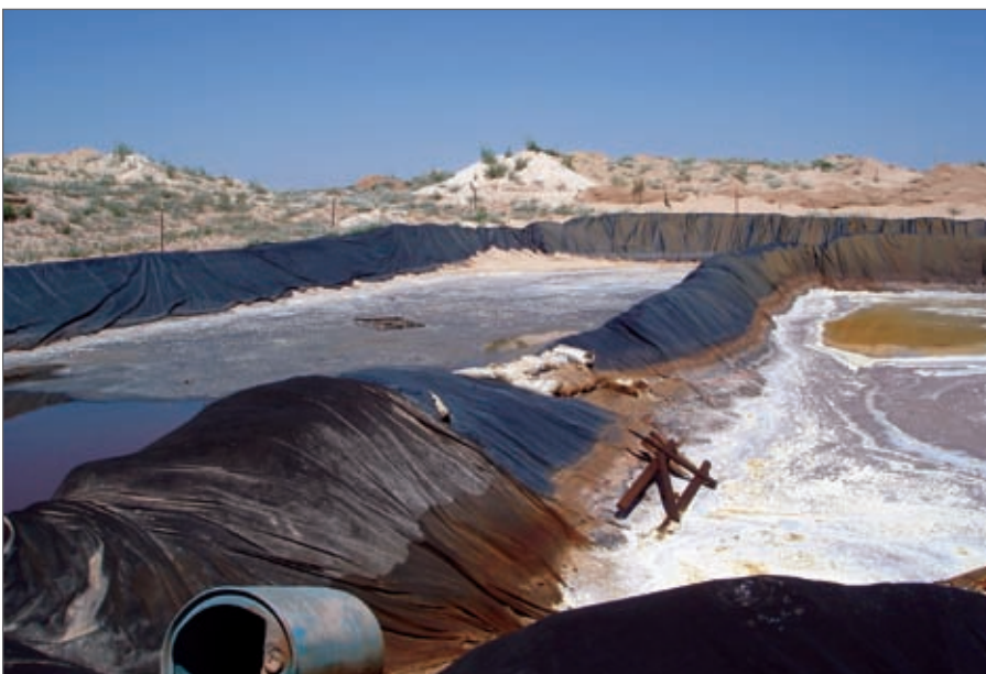
Double horseshoe reserve pits retain cuttings for their eventual disposal. They also hold various fluids such as brines and fresh water. Breached liners can result in contamination of the subsoil or underground aquifer.
