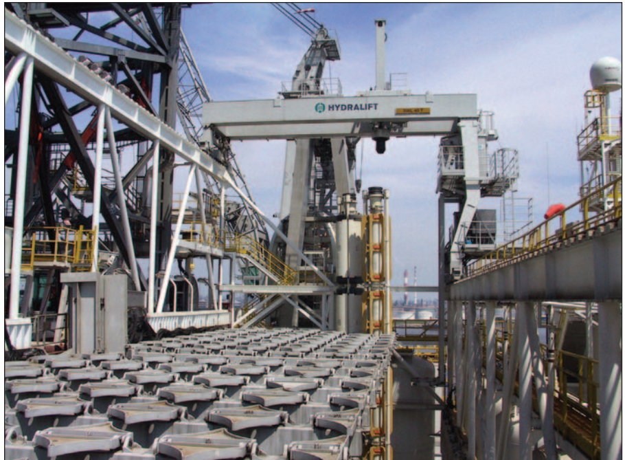
The riser gantry crane is used to transfer tubulars between the rig floor and the riser setback area, which can accommodate 100 joints of 75 ft riser stored vertically.
